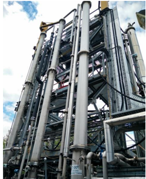
Figure 2: CO 2 capture plant
